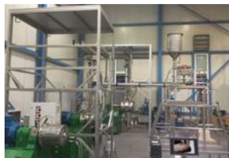
Fig. 1 Powder manufacturing installations at Zoz
